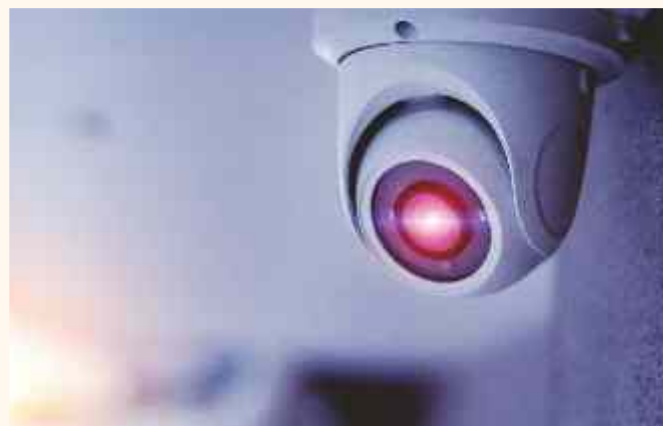
CCTV for Common Area
