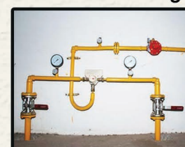
Central LPG Station.
