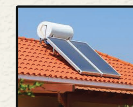
Solar Power for hot water.
