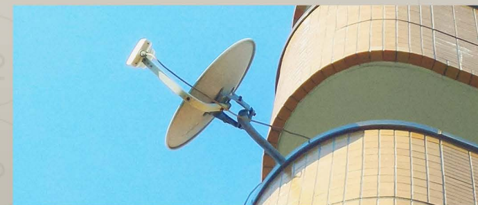
Common DTH Facility
